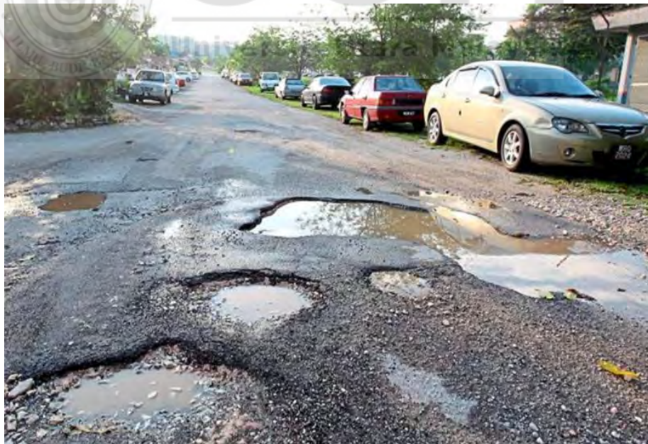
(Figure 2.2.2 Road potholes)
